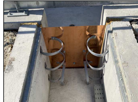
Fig. 4. Copper termination plates.
