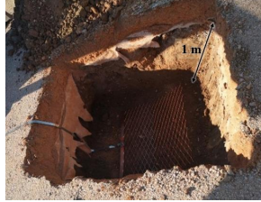
Figure 6: Grounding point created for the equipment.
